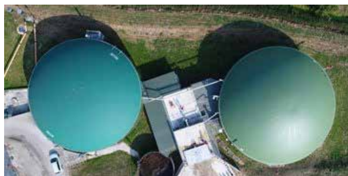
Biogas plant in Bentzin (District of Vorpommern-Greifswald). The plant will use a combination of ultrasonic and plasma treatment to increase the disintegration of processed biomass substrates and thus ultimately the biogas yield.
